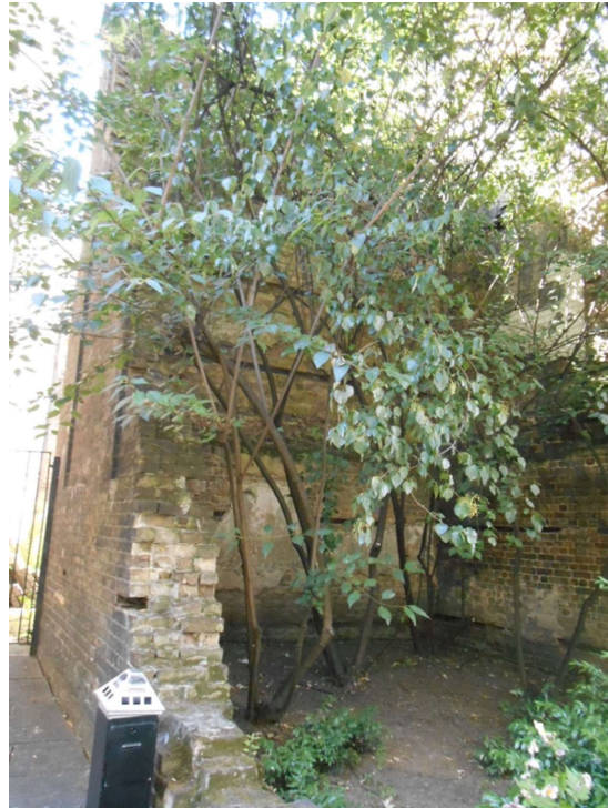
Churchyard site is adjacent to the London Wall, and this will require careful consideration
